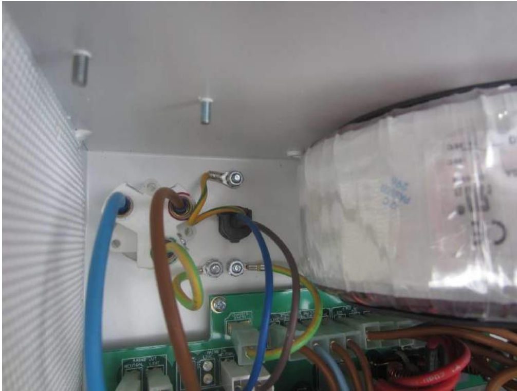
Fig 17: Supply cord entry and rear of socket outlet after test
