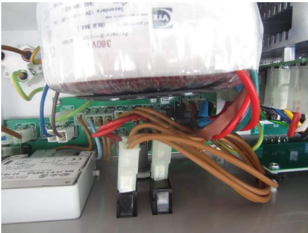
Fig 20: Switches after test
