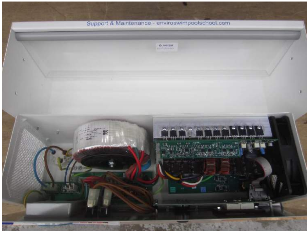
Fig 16: Internal component after test
