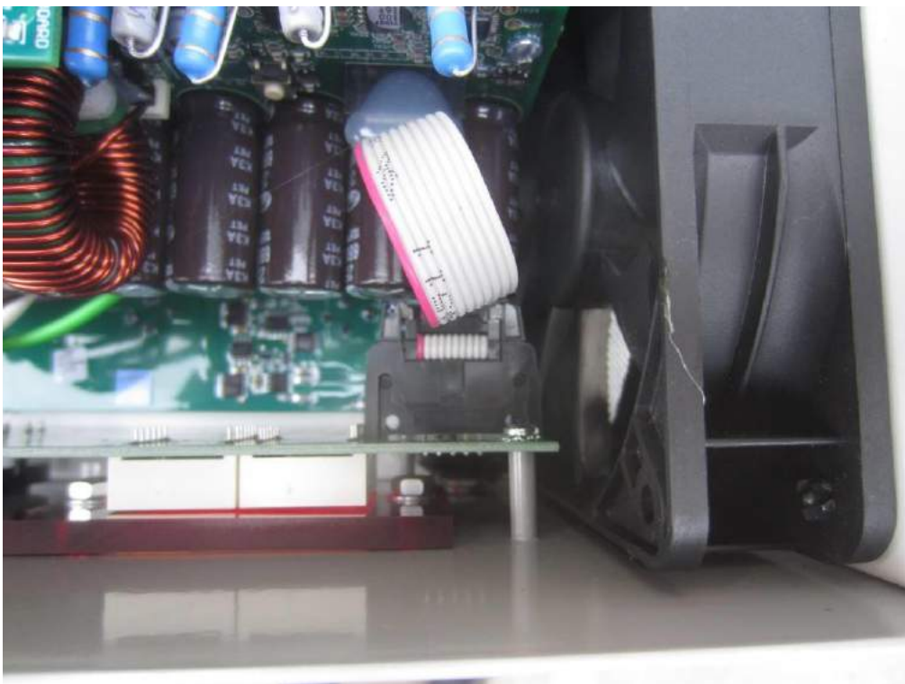
Fig 22: Thermo fan assembly after test
