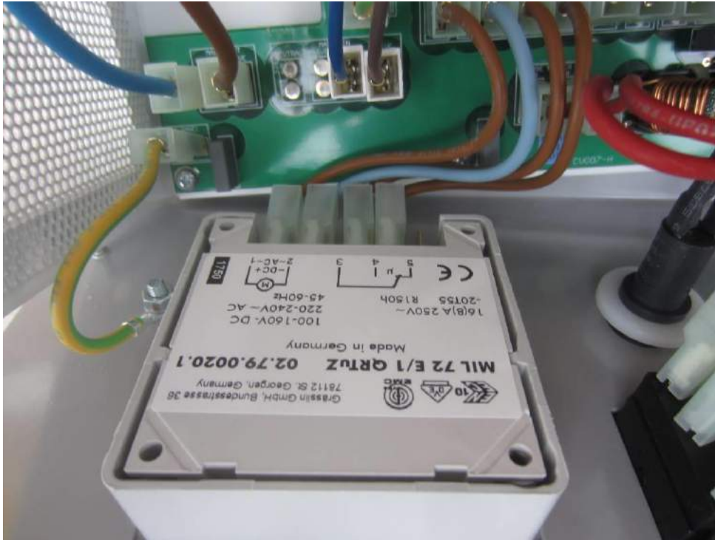
Fig 19: Timer connections after test
